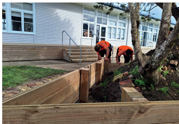
Students from the Building Academy built a retaining wall around the school. Photo credit: Bay of Islands College
